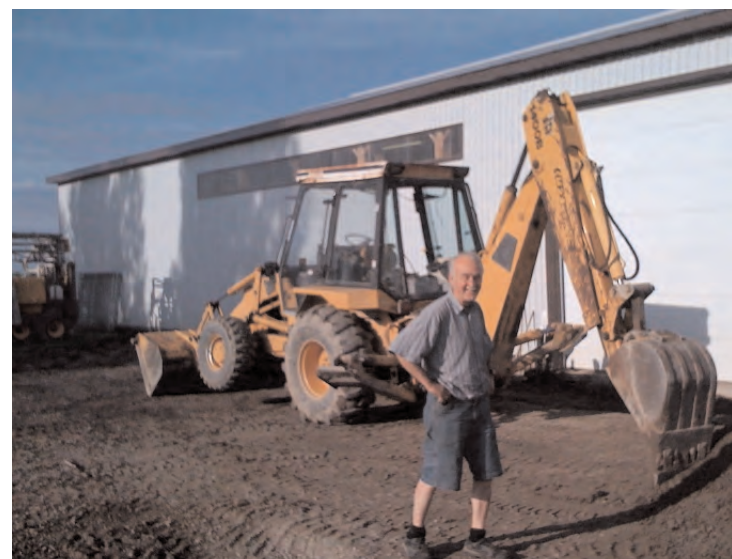
John Digs His New Pad. This is where the six new stainless steel tanks will be placed.
